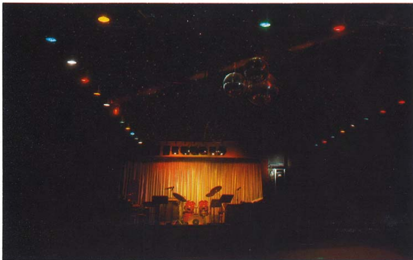
Fibre optic ceiling recently installed by Northern Lights at the Regency Club in Morecambe.
