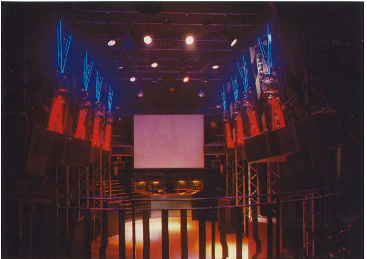
A view across the dance floor of Joe Paparazzi's in Glasgow, showing the lighting panels in their store position with video screen in use.
